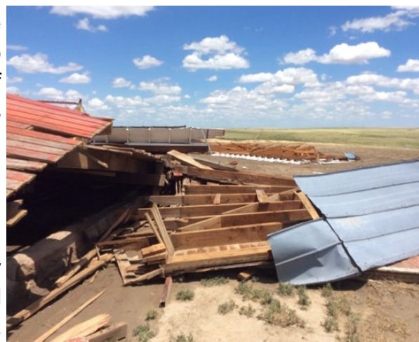
Straight-line wind damage in Cheyenne County.
